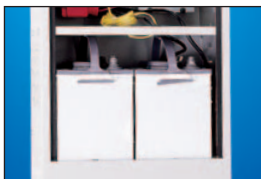
two batteries (deep cycle) can be accommodated in the cabinet
