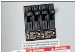
circuit breakers six 20-amp branch breakers provide protection for the external loads
