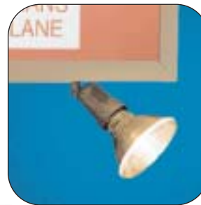
150 watt flood lamp illuminates spikes
