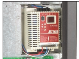
variable speed motor drive
